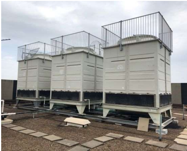
Picture: Cooling Towers
