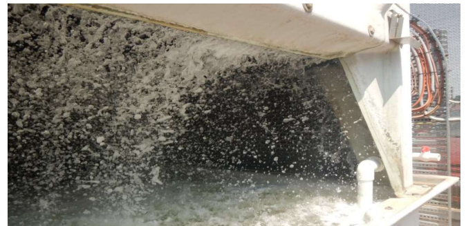
Picture: Inside a cooling tower
